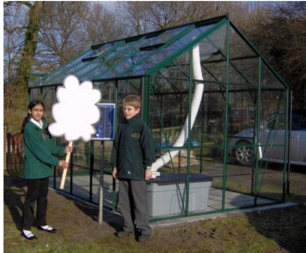
Heater in place with hose outlet taken to apex of greenhouse
